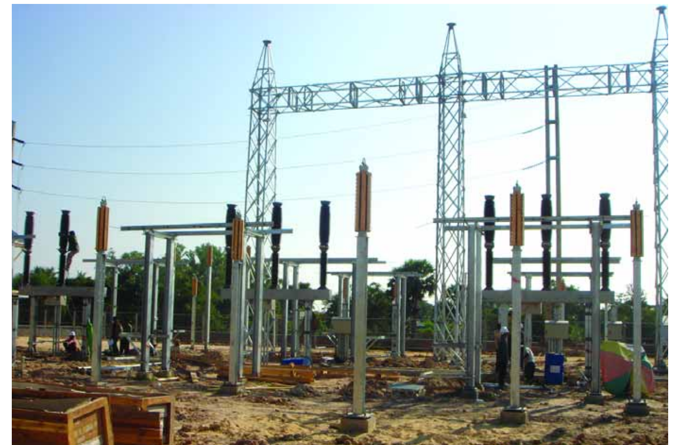
A power sub-station funded with a loan from FTB
